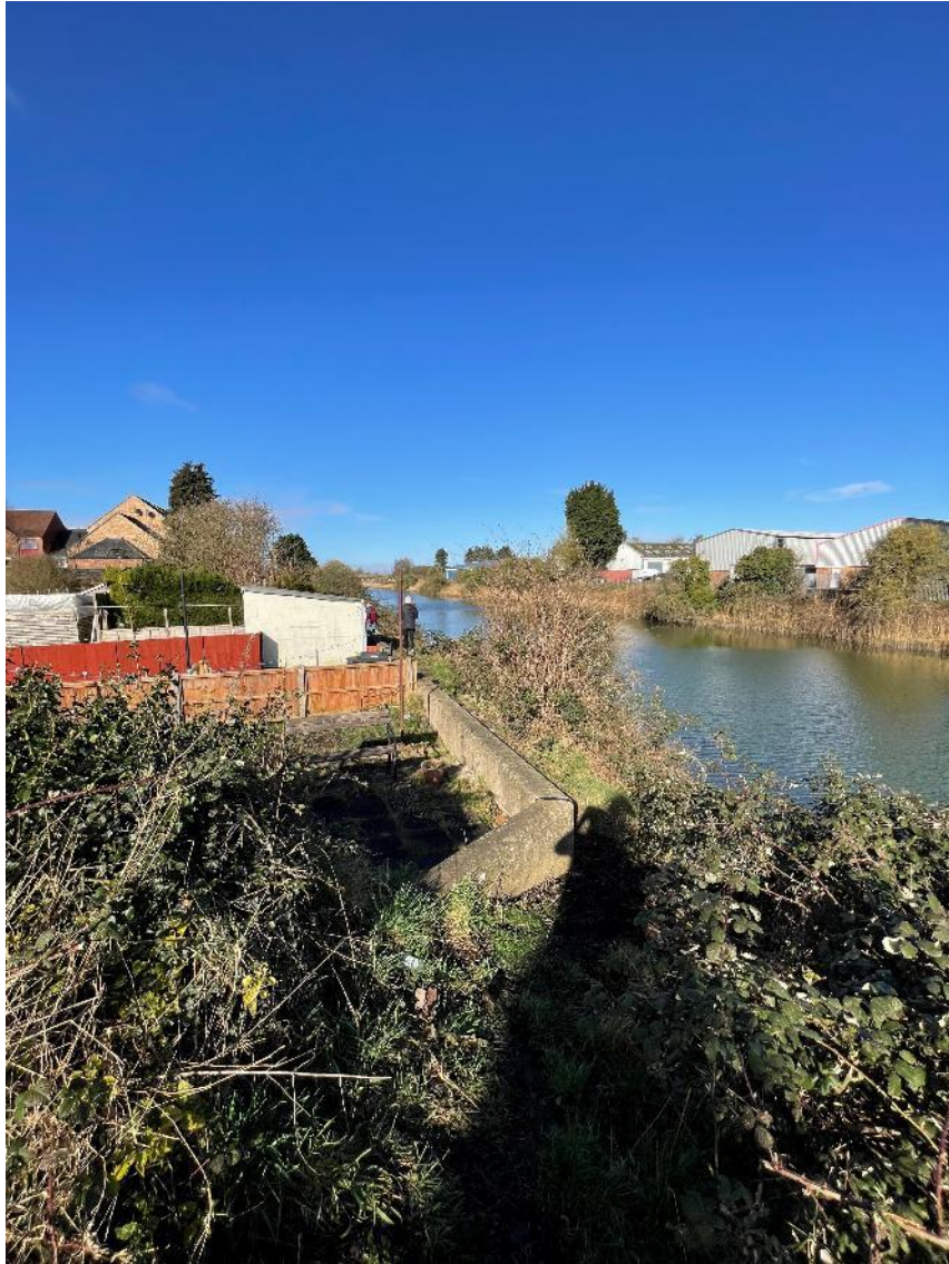
(Photograph 2 – Western section of EA flood wall along the southern bank of the SFFD; facing west)
