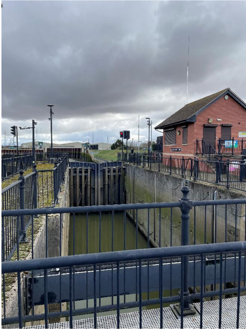
(Photograph 13 – Sluice gate, also used as a navigational lock, at Black Sluice Complex; facing east)
