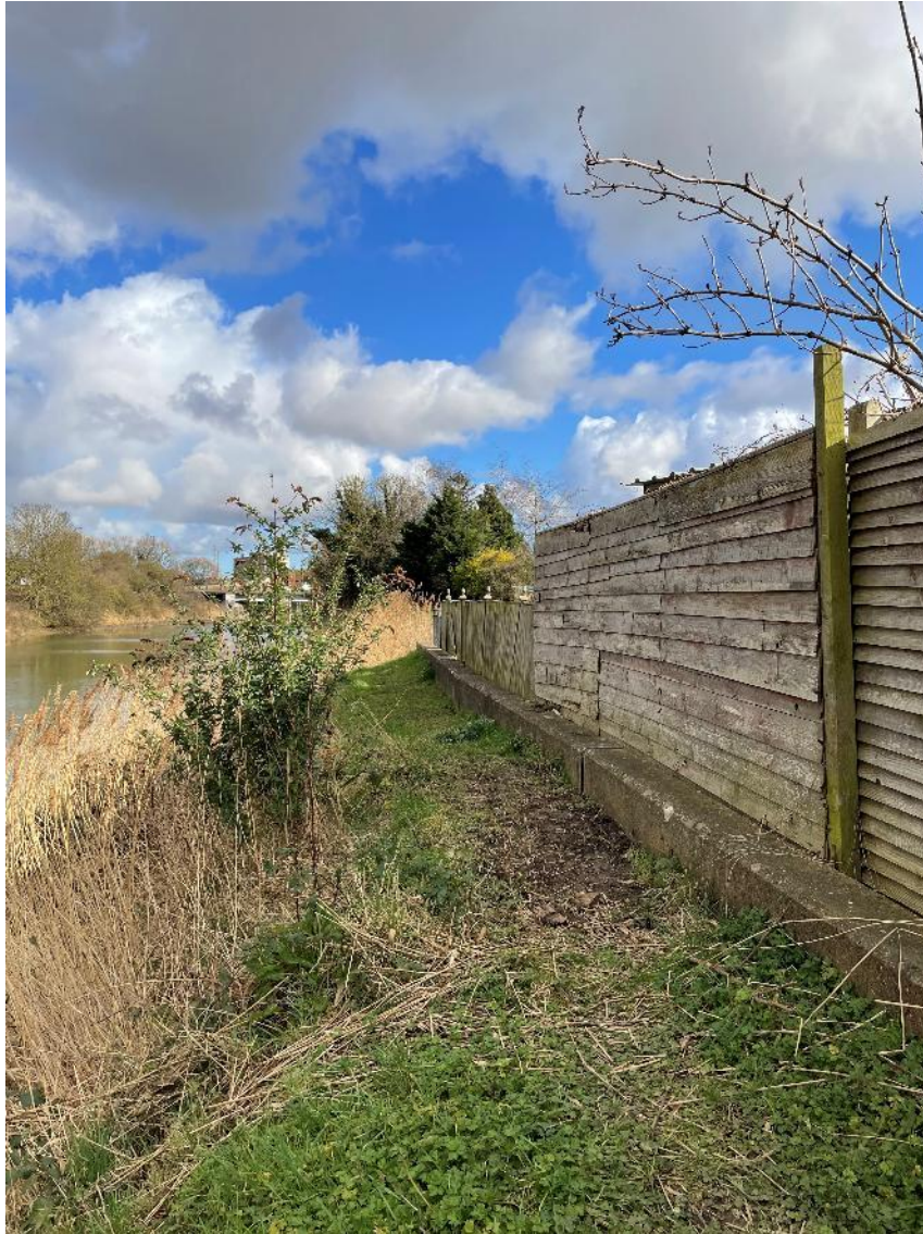
(Photograph 3 – Eastern section of EA flood wall along the southern bank of the SFFD; facing east)
