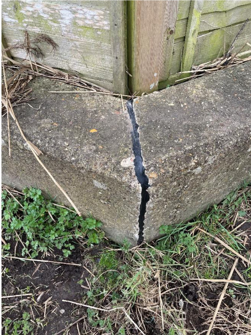
(Photograph 4 – Replaced seal on the eastern section of flood wall along the SFFD)
