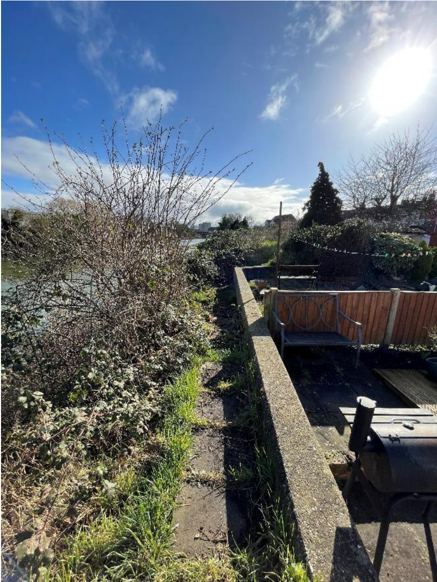
(Photograph 1 – Western section of EA flood wall structure along the southern bank of the SFFD; facing east)
